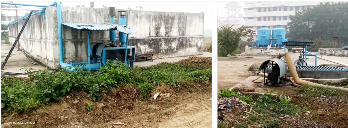
Plate 4: Sep in the premises
